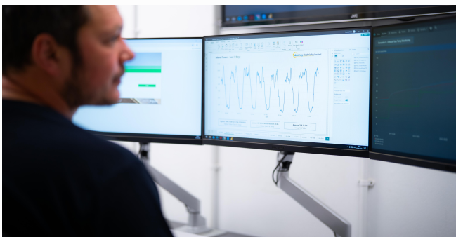
Alderney Power Station Controls.
